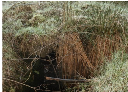
300Ø HDPE pipe outlet
