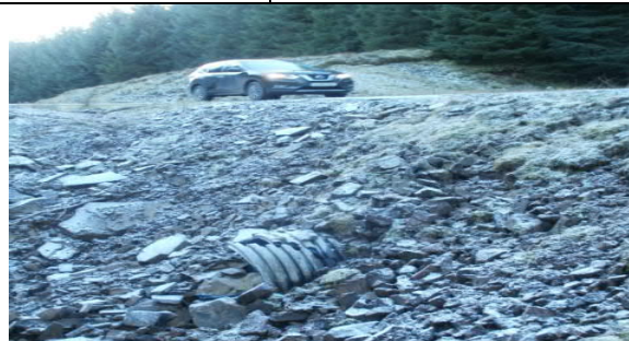
Damaged 450Ø HDPE pipe outlet to be replaced
